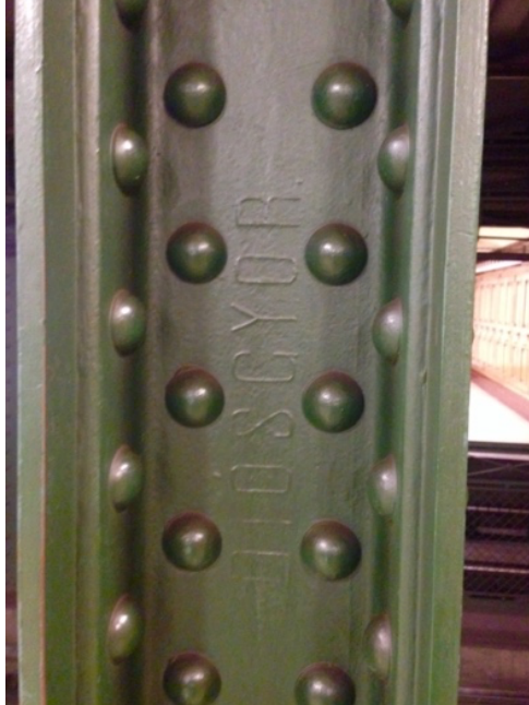
FIGURE 2. Imprint of the Diósgyőr Steel Works on a Supporting Beam of the Millennium Underground Railway
